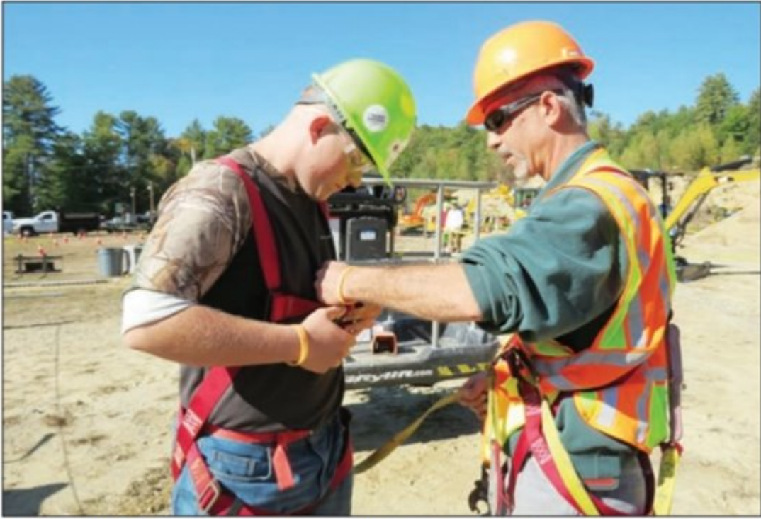
CJ Drabble (left) puts on a safety harness before operating the lift with a member of the Bow, NH, DPW.
